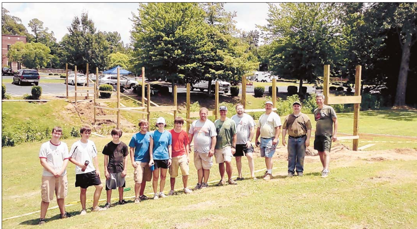
Bill Fielder (from left), James Chapman, Logan Walker, Allan Sisson, Jennifer Sisson, Jonathan Chapman, Joey Markham, Larry Sisson, Jon Pace, Paul Hayes, Barry Chapman and Jerry Sisson construct a wooden structure that will be the foundation of the new bridge that connects Germantown Church of Christ to Friendship Park.
